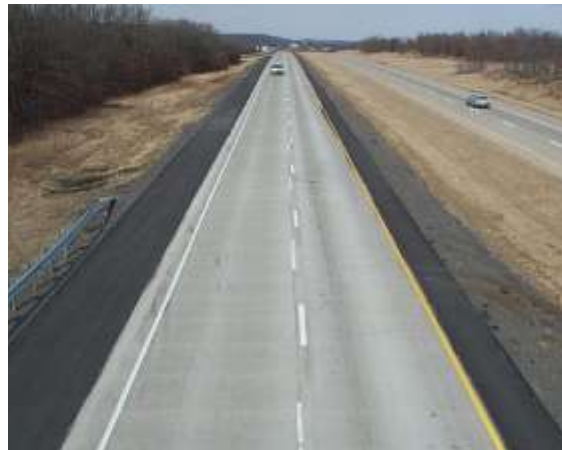
Whitetopping is gaining in popularity in fixing deteriorating hot-mix asphalt pavements and includes the benefit of having a higher albedo, better performance and increased durability over asphalt.
