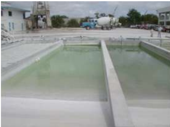
Water settling basins separate solids from water and allow for the recycling of waste and wash water at concrete plants.
