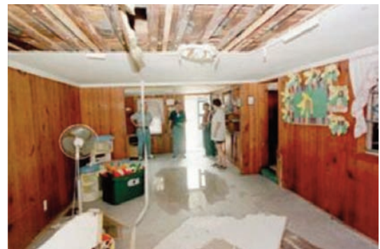
Source: Federal Emergency Management Agency, photograph taken by Dave Gatley of FEMA. Moisture damage is not just related to flooding. Here, an inspector is seen evaluating water damage when a roof was compromised by wind and rain.
