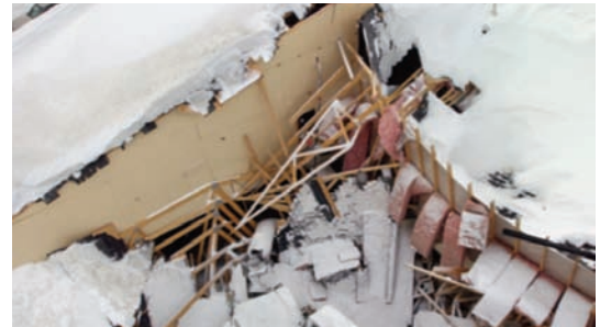
Source - Institute for Business and Home Safety In many instances roof collapse due to snow loads not only results in damage to roof and building contents below but may also remove lateral support, allowing walls to collapse.
