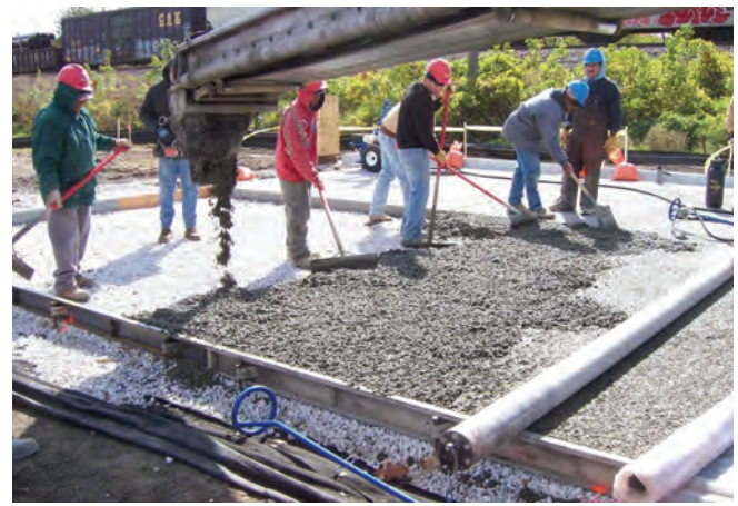
Figure 3.7 Pervious concrete being placed (photo courtesy of John Kevern, University of Missouri-Kansas City)
