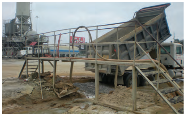
Figure 5.8 Washout pit used to clean concrete trucks (photo courtesy of Gary Fick, Trinity Construction Management, Inc.)
