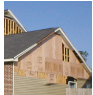
Damage to siding and sheathing as a result of high winds.
