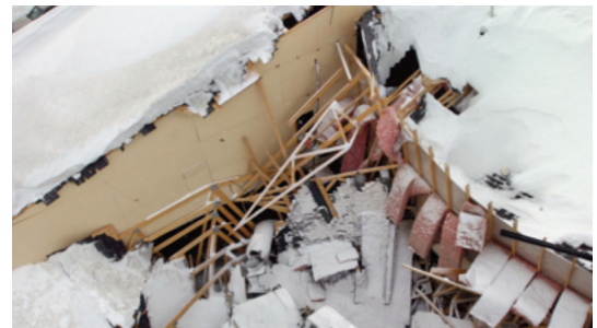
Source - Institute for Business and Home Safety In many instances roof collapse due to snow loads not only results in damage to roof and building contents below but may also remove lateral support, allowing walls to collapse.
