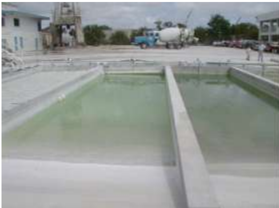
Water settling basins separate solids from water and allow for the recycling of waste and wash water at concrete plants.
