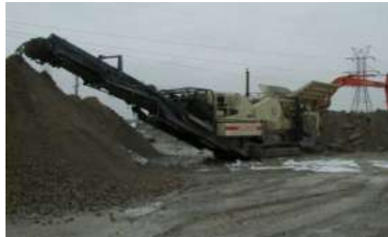
Crushing concrete and then using the material for aggregate is an opportunity to qualify for recycled content credit.
