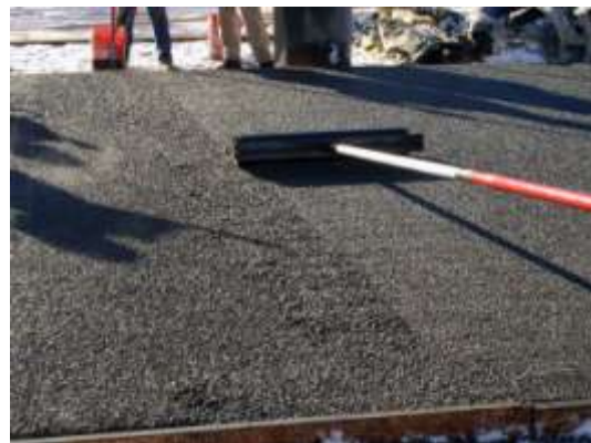
Pervious concrete finishing uses similar equipment as for finishing standard concrete; technique is the key.
