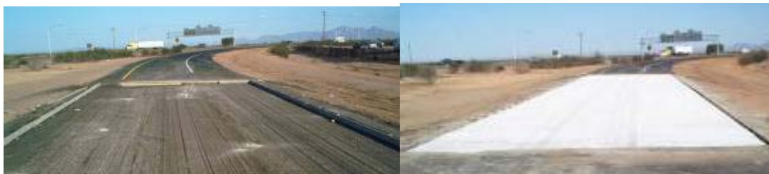
Figure 8 A thin white topping project in Phoenix: (a) grinding down the existing asphalt base, and (b) curing the final surface. Photos courtesy of National Center of Excellence, Arizona State University.
